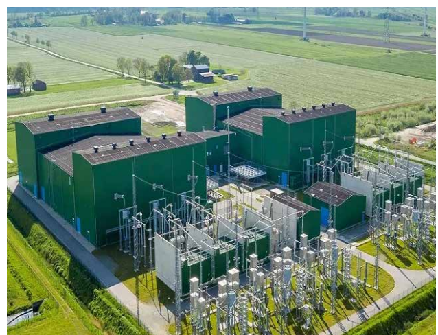
Figure 32. HVDC Converter Station (Hitachi Energy [27])
