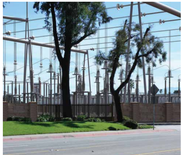
Figure 9. 500kV Transition Station, Chino Hills (Southern California Edison)
