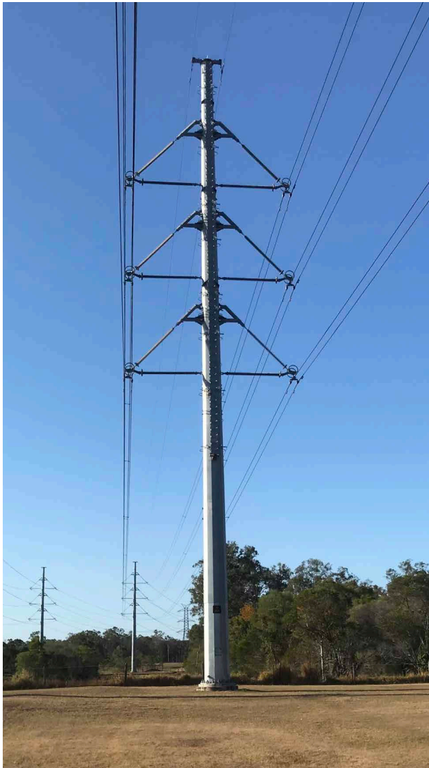
Figure 6. 275kV Double Circuit Compact Steel Pole
