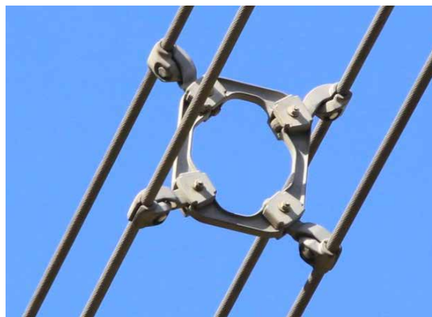
Figure 2. Transmission Line Quad Bundled Conductor with Spacer (Marcus Wong)
