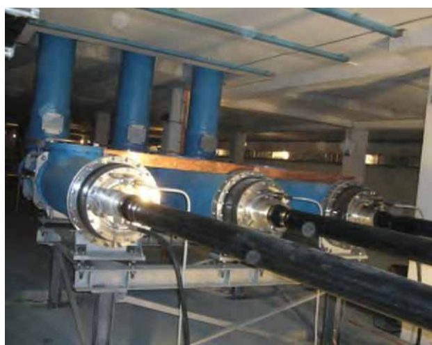
Figure 19. Typical HV Gas Insulated Switchgear (GIS) with cable terminations Installed in Horizontal Position (Nexans / Frederic Lesur)
