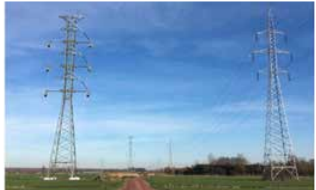
Figure 5 – Example of the tower for the compact 380 kV overhead line equipped with insulated cross-arms based on composite insulators (left) in parallel with the existing 150 kV line (right) [23]
