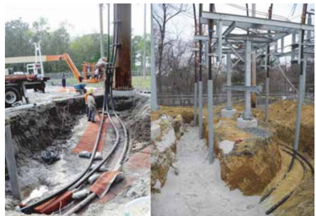
Figure 28 Direct buried section near a compact transition pole with one cable per phase (left) and conventional risers with two cable per phase (right) [31]
