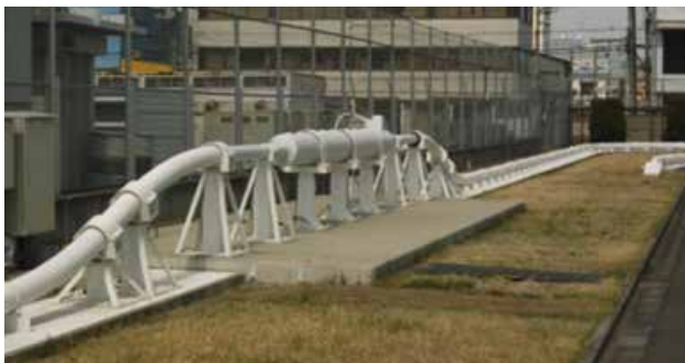
Figure 24 TEPCO AC HTS cable with a joint at Asahi substation in Yokohama/Japan [52]
