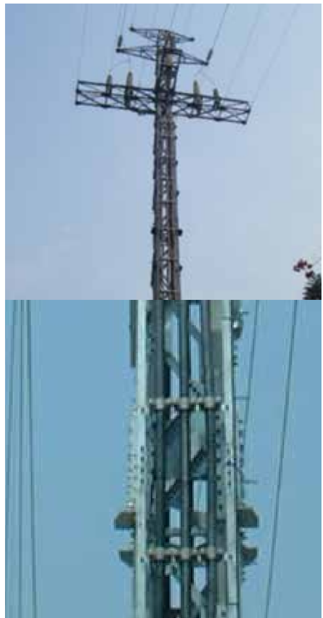
Figure 30 Junction tower with structural steel (left) and lateral view of flat arrangement of cables (right) [50]
